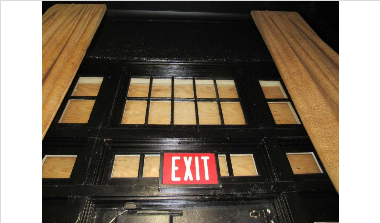
Photo #32 Gulfstream Hotel Building 1 Lake Ave, Lake Worth, FL 33460 Close-up of original exit doors in east wing (boarded from exterior) (11/7/2019)
