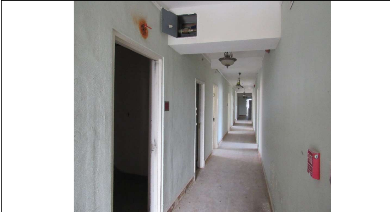
Photo #54 Gulfstream Hotel Building 1 Lake Ave, Lake Worth, FL 33460 Northwest view of first floor interior (7/10/2020)
