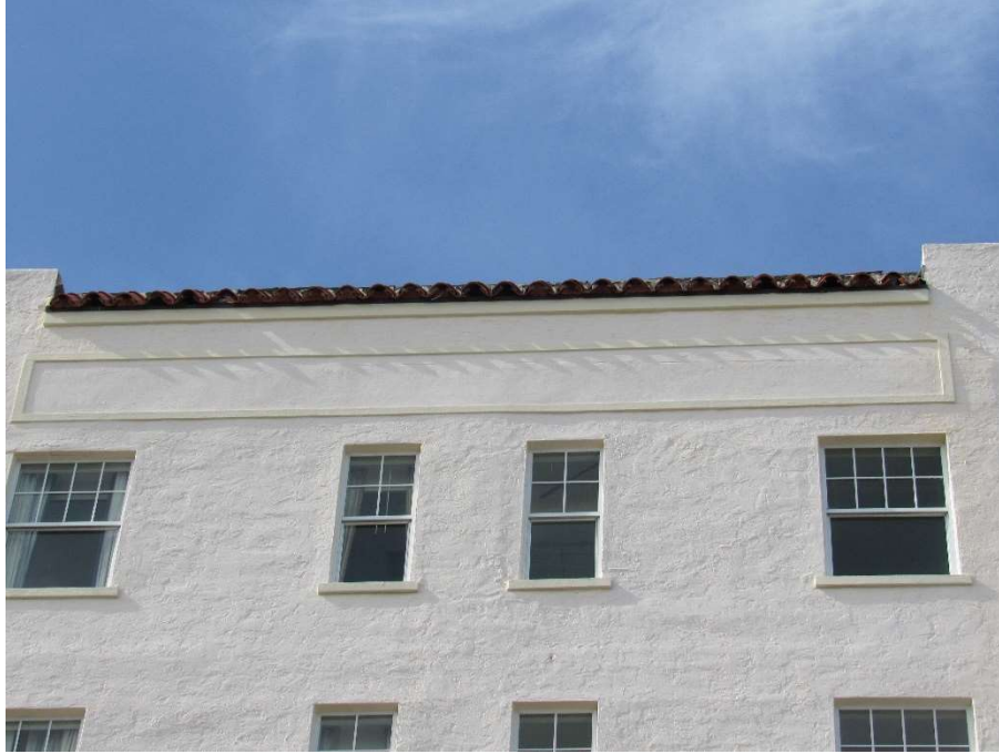
Photo #15 Gulfstream Hotel Building 1 Lake Ave, Lake Worth, FL 33460 Windows and terracotta roofing N elevation (3/20/2020)
