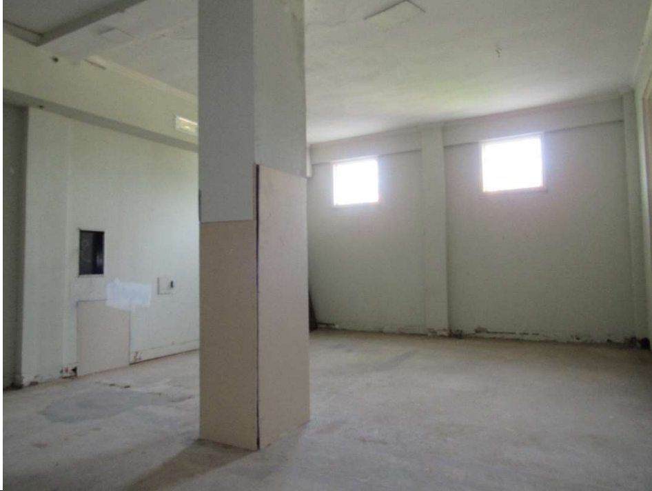
Photo #25 Gulfstream Hotel Building 1 Lake Ave, Lake Worth, FL 33460 Front room facing SW (7/10/2020)
