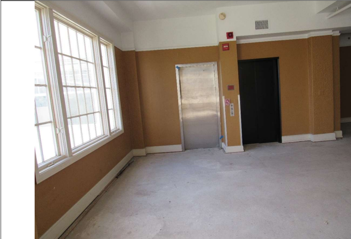
Photo #43 Gulfstream Hotel Building 1 Lake Ave, Lake Worth, FL 33460 Mezzanine elevator lobby (7/10/2020)
