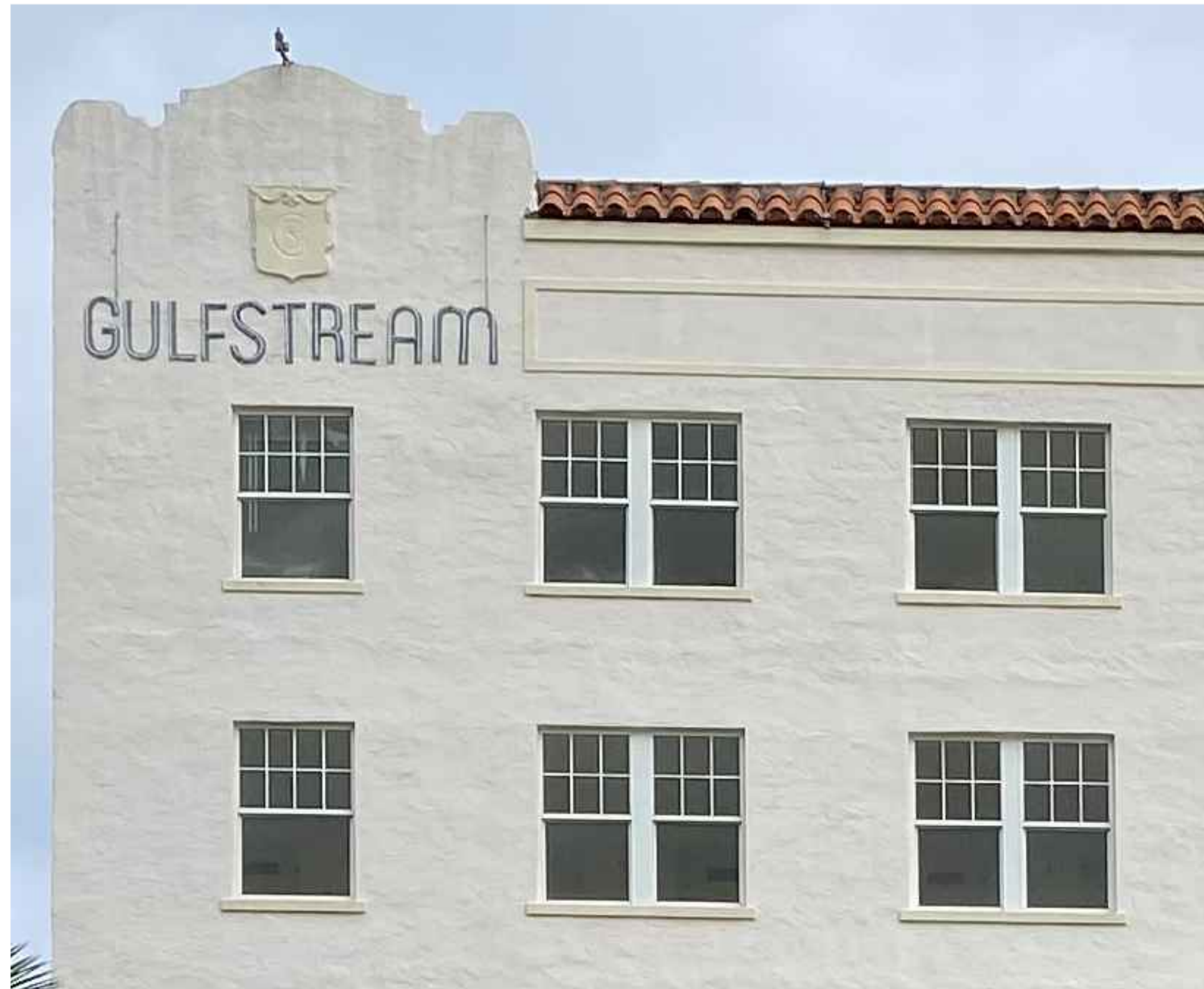
TRIMS CLAY BARREL TILE ROOF GULFSTREAM SHIELD AND SIGNAGE EXISTING WINDOWS TO BE REPLACED WITH NEW WINDOWS (MULLION CONFIGURATION TO MATCH EXISTING)
