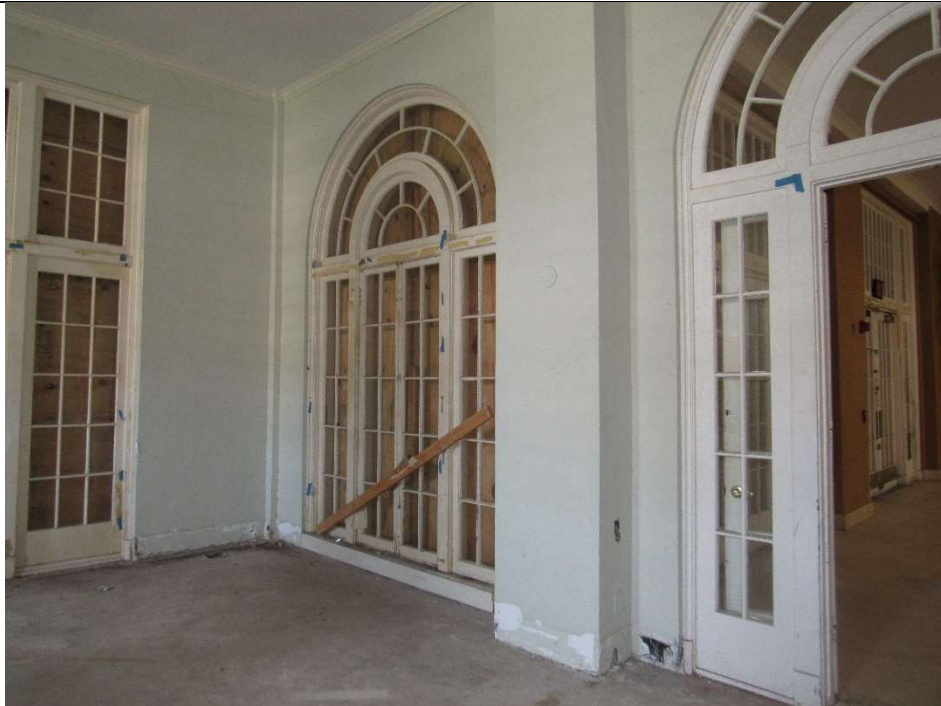
Photo #24 Gulfstream Hotel Building 1 Lake Ave, Lake Worth, FL 33460 Front room facing NE (7/10/2020)
