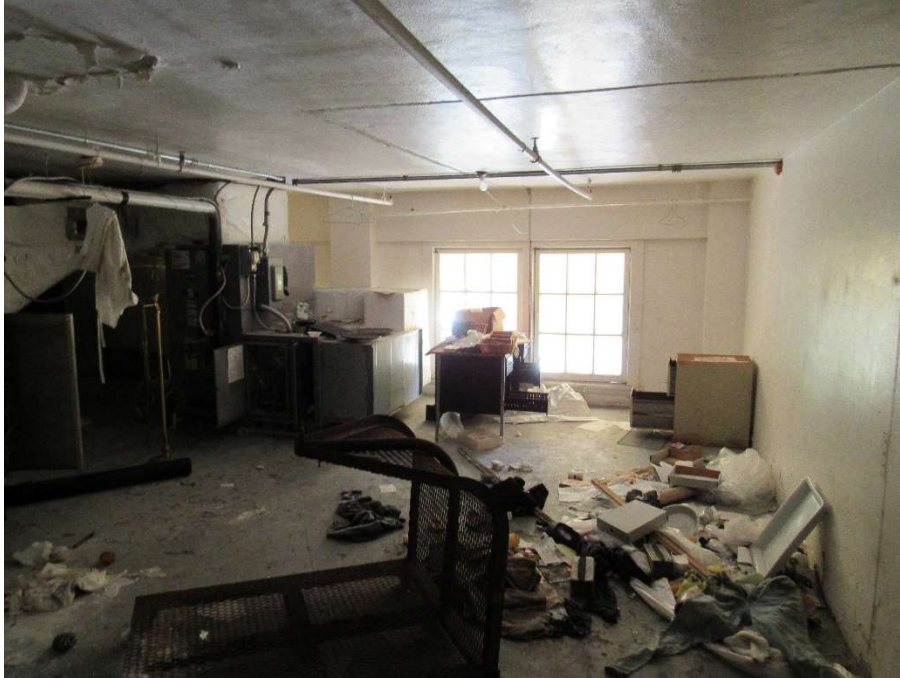
Photo #40 Gulfstream Hotel Building 1 Lake Ave, Lake Worth, FL 33460 Mechanical 2 (7/10/2020)
