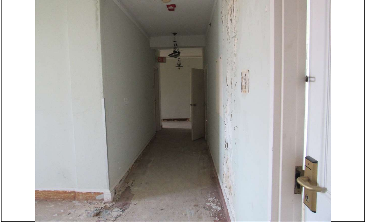
Photo #70 Gulfstream Hotel Building 1 Lake Ave, Lake Worth, FL 33460 Sixth floor corridor (7/10/2020)
