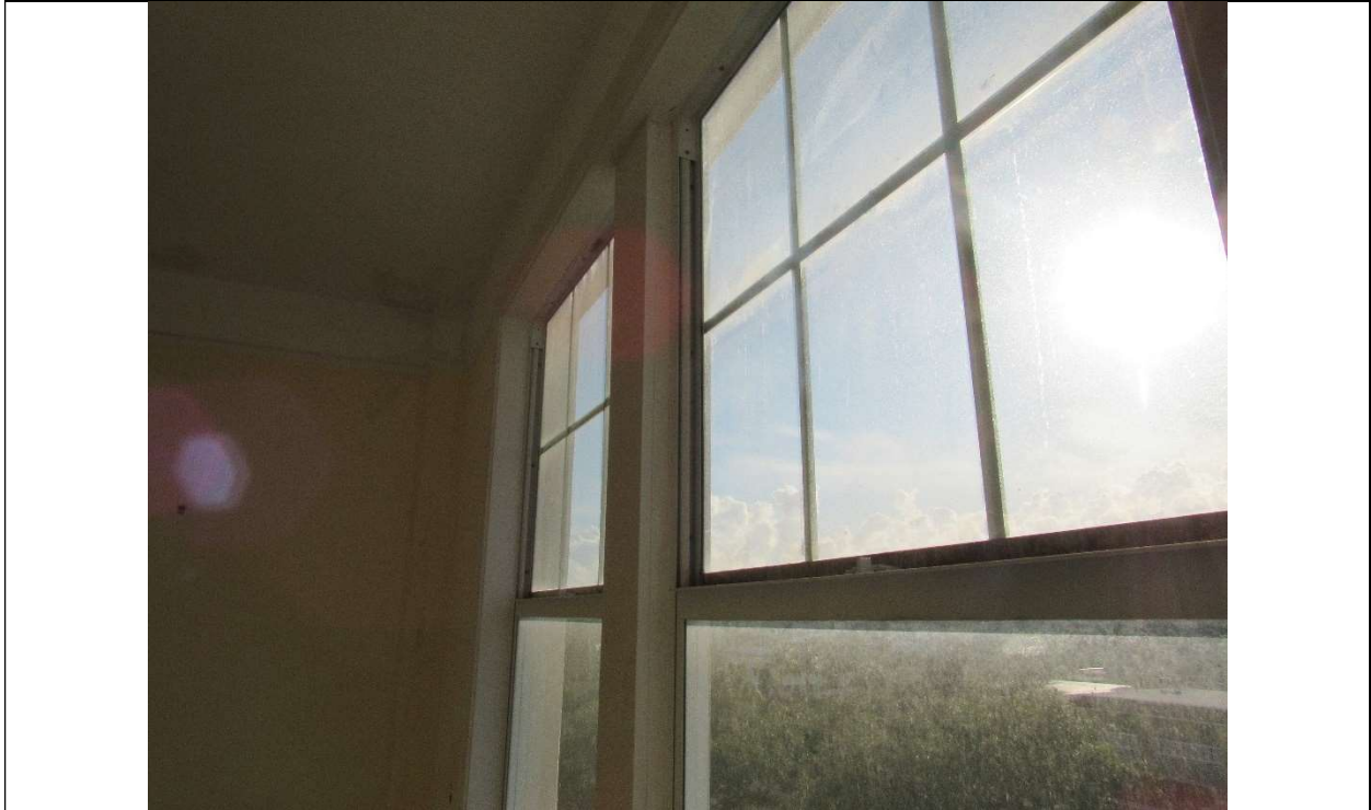
Photo #60 Gulfstream Hotel Building 1 Lake Ave, Lake Worth, FL 33460 Close-up of window (7/10/2020)
