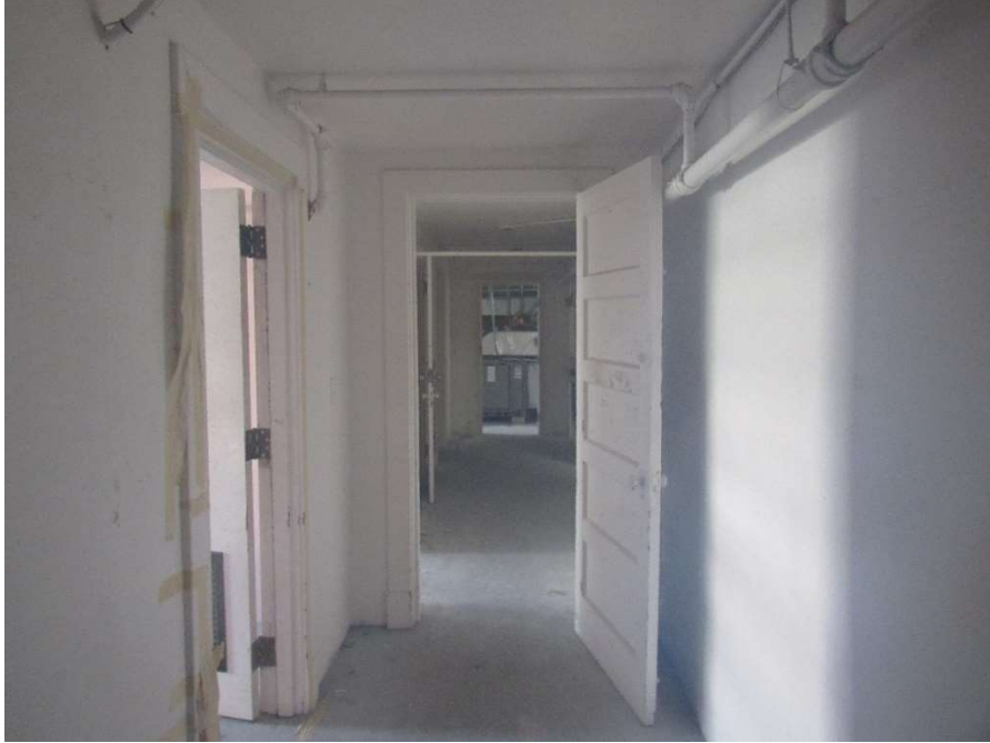
Photo #38 Gulfstream Hotel Building 1 Lake Ave, Lake Worth, FL 33460 Mechanical hallway (7/10/2020)
