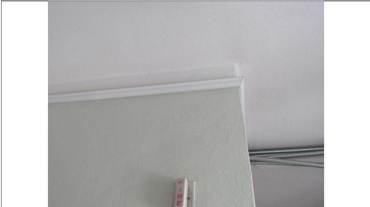
Photo #55 Gulfstream Hotel Building 1 Lake Ave, Lake Worth, FL 33460 Close-up of crown molding – third floor (7/10/2020)
