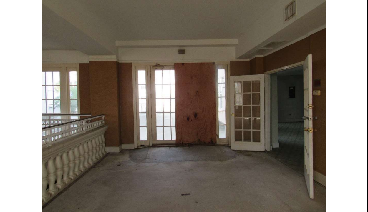
Photo #44 Gulfstream Hotel Building 1 Lake Ave, Lake Worth, FL 33460 Northwest view of basement interior NW (7/10/2020)
