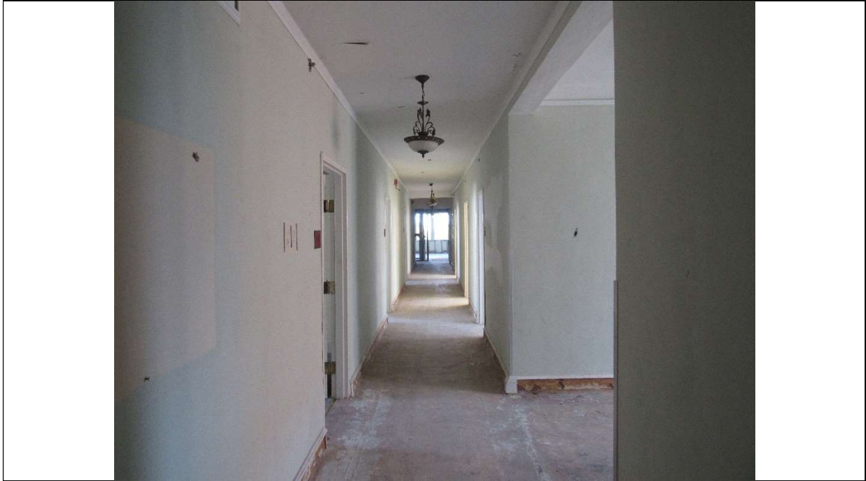
Photo #52 Gulfstream Hotel Building 1 Lake Ave, Lake Worth, FL 33460 Third floor corridor (7/10/2020)
