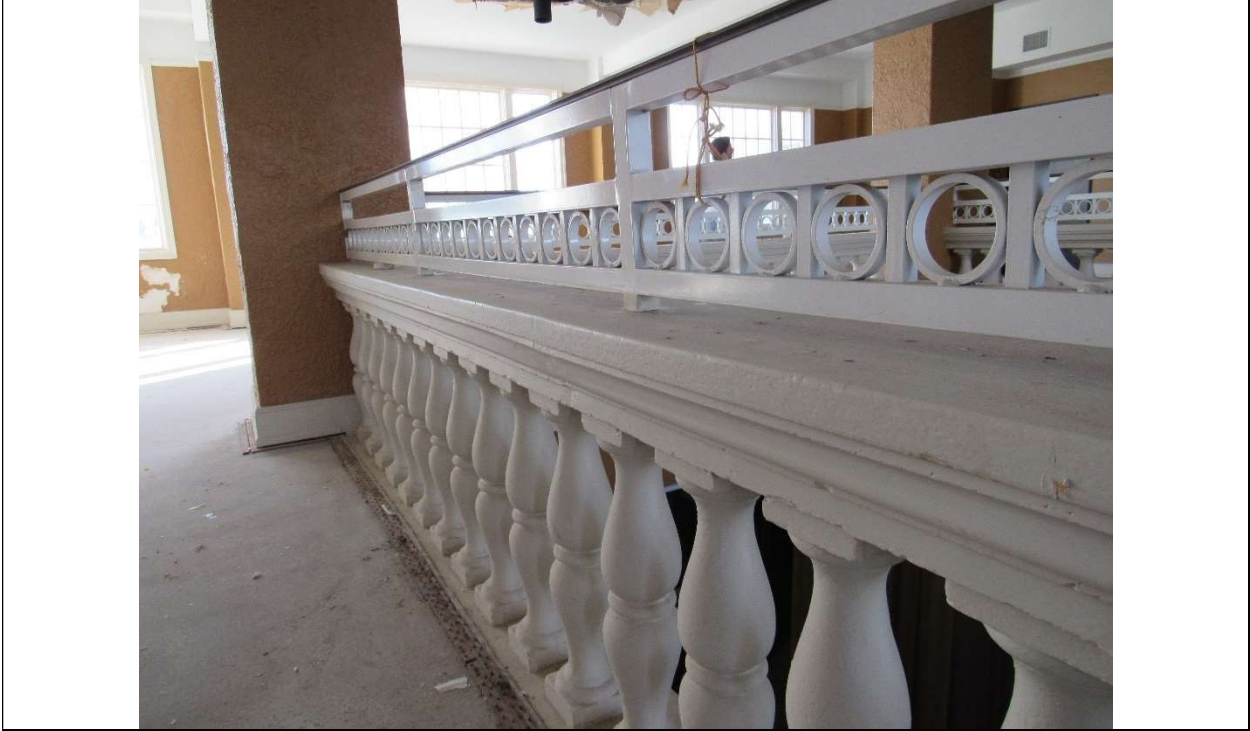
Photo #42 Gulfstream Hotel Building 1 Lake Ave, Lake Worth, FL 33460 Close-up of mezzanine balcony (7/10/2020)
