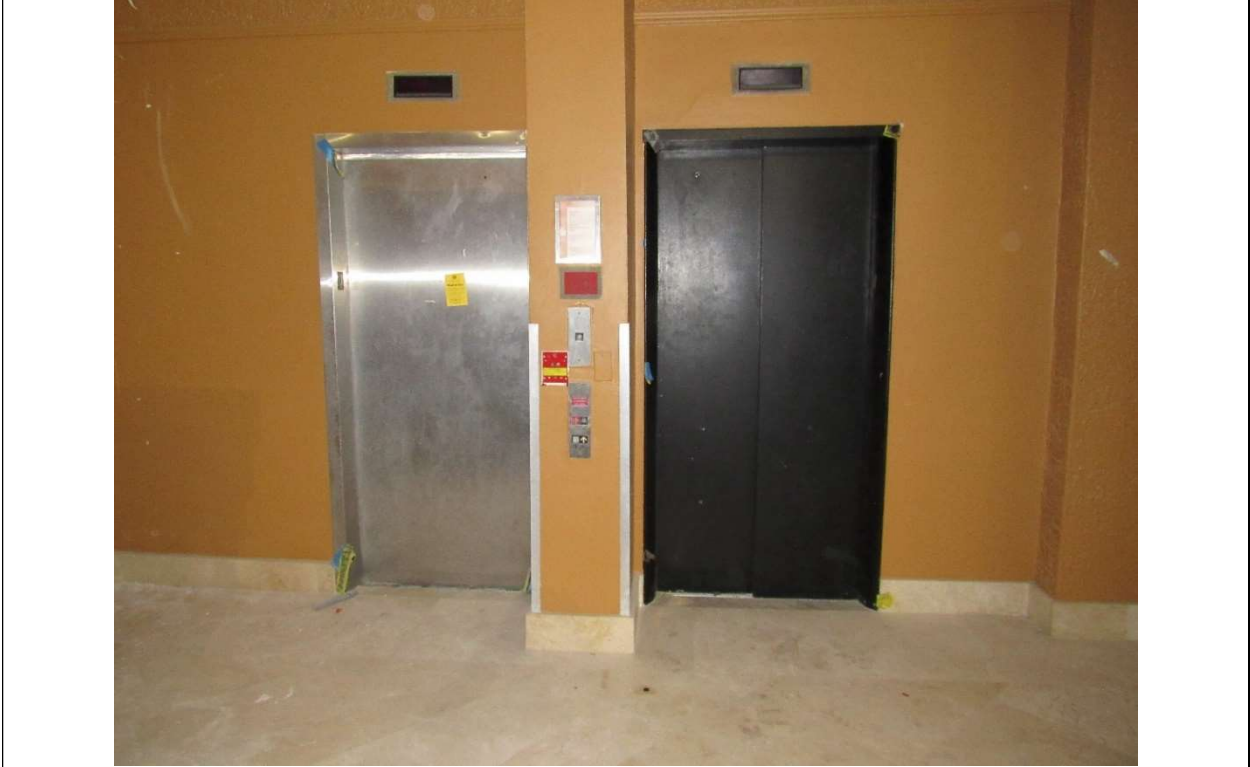
Photo #21 Gulfstream Hotel Building 1 Lake Ave, Lake Worth, FL 33460 Existing elevators in lobby (11/7/2019)
