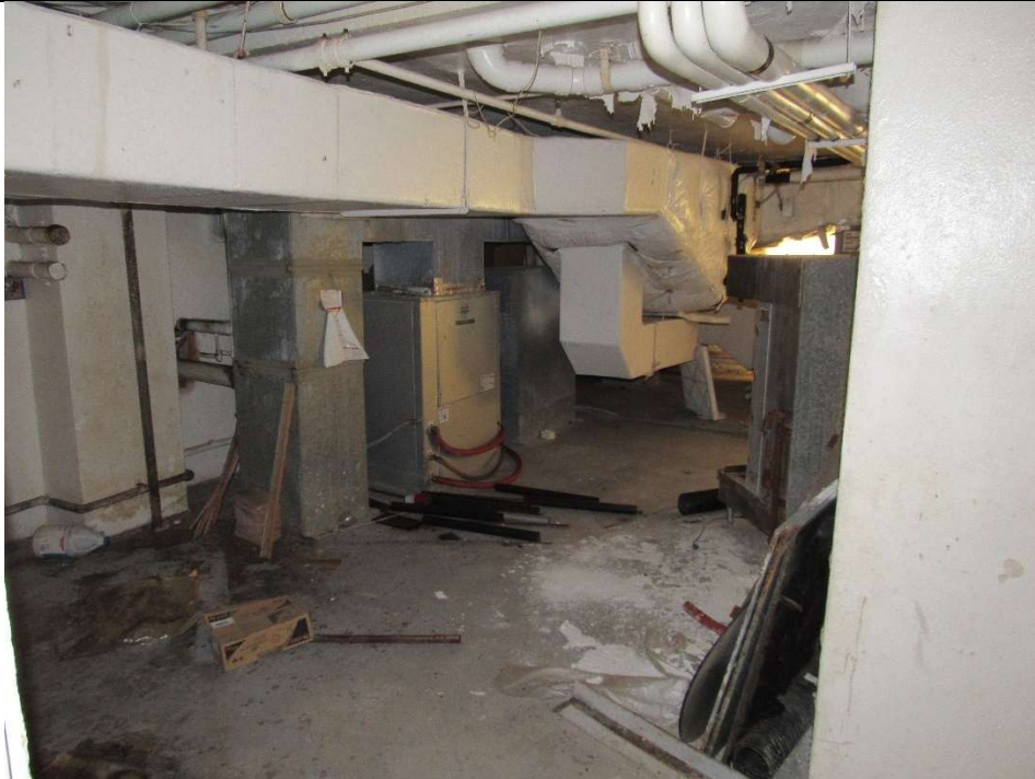
Photo #39 Gulfstream Hotel Building 1 Lake Ave, Lake Worth, FL 33460 Mechanical (7/10/2020)
