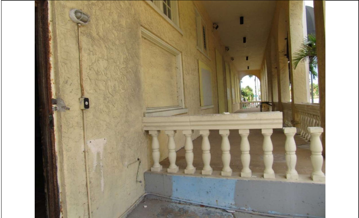
Photo #11 Gulfstream Hotel Building 1 Lake Ave, Lake Worth, FL 33460 Interior of colonnade E elevation (3/12/2020)
