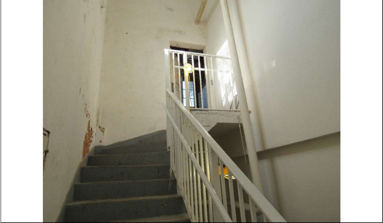
Photo #74 Gulfstream Hotel Building 1 Lake Ave, Lake Worth, FL 33460 Stairwell to rooftop (7/10/2020)
