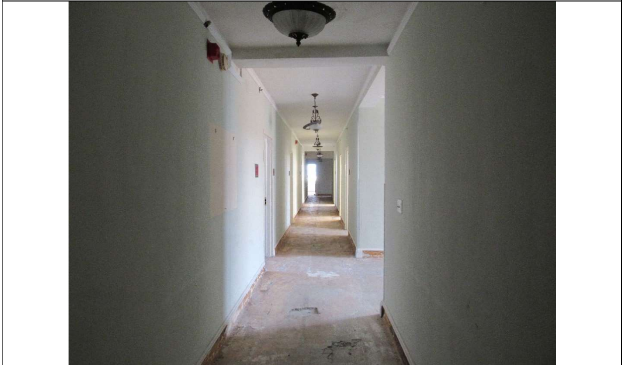
Photo #63 Gulfstream Hotel Building 1 Lake Ave, Lake Worth, FL 33460 Fifth floor corridor (7/10/2020)
