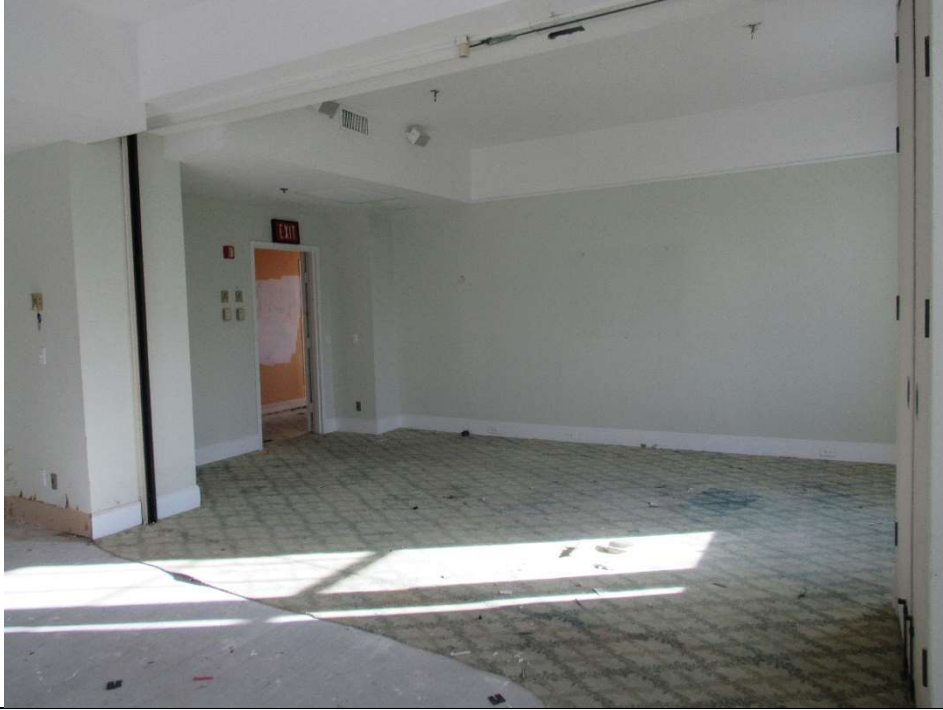
Photo #50 Gulfstream Hotel Building 1 Lake Ave, Lake Worth, FL 33460 2 nd floor room (7/10/2020)
